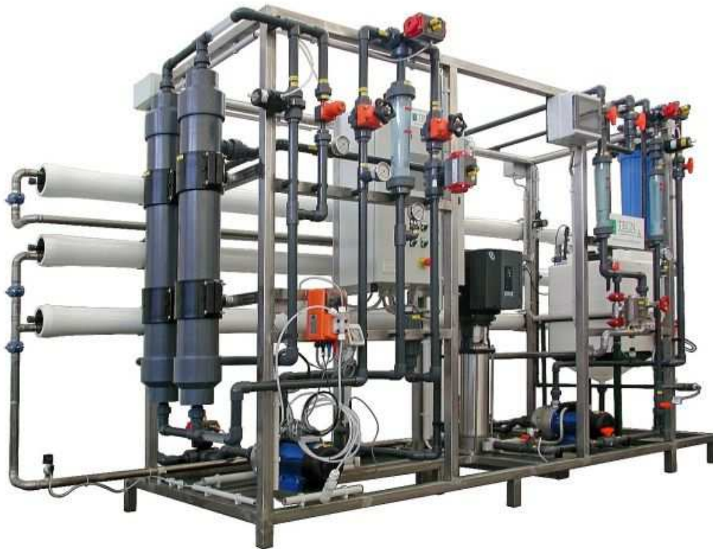
UF combined on RO skid
