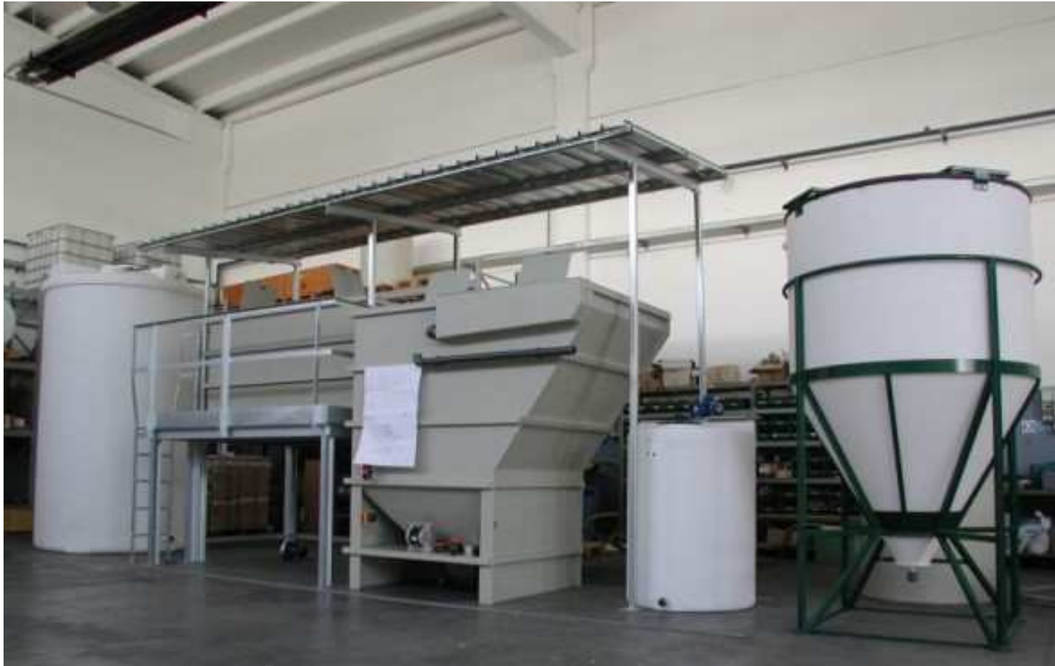
Chemical-physical plant - 7 m 3 /h
