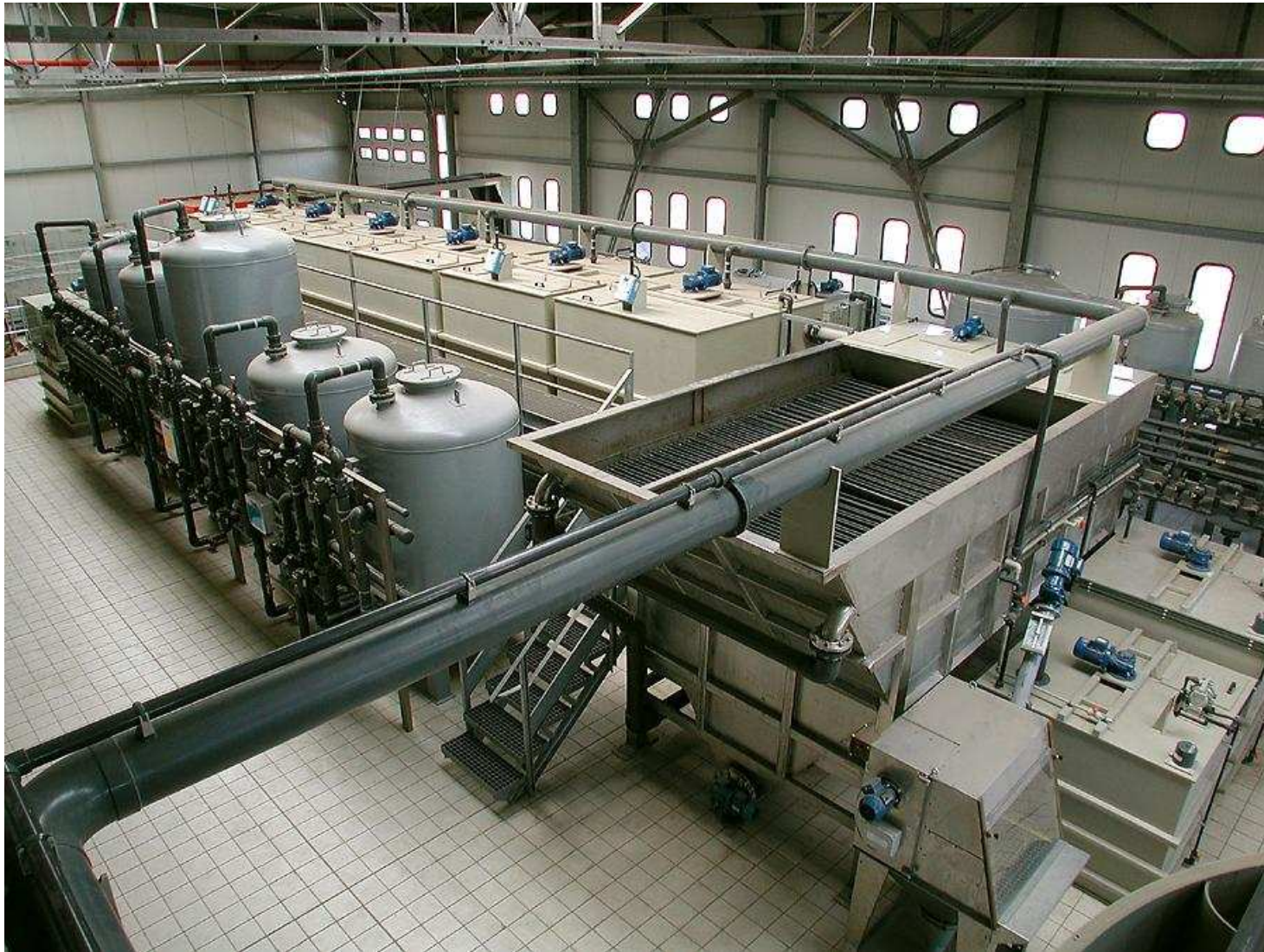
Chemical-physical plant 20 m 3 /h, with reaction sections (Fenton, sulfide and basification)
