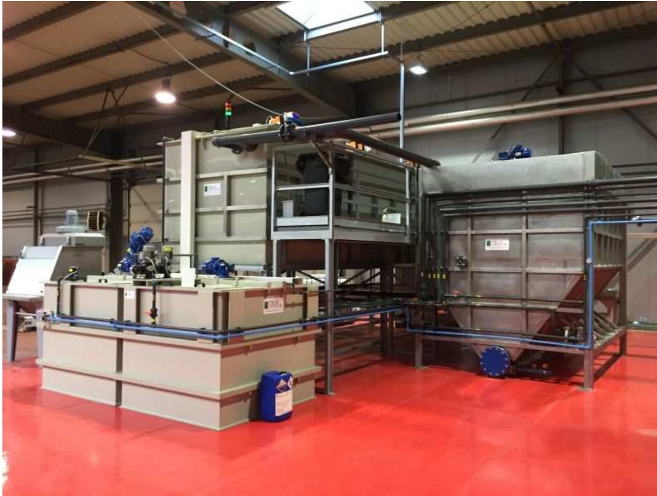
Chemical-physical plant 20 m 3 /h
