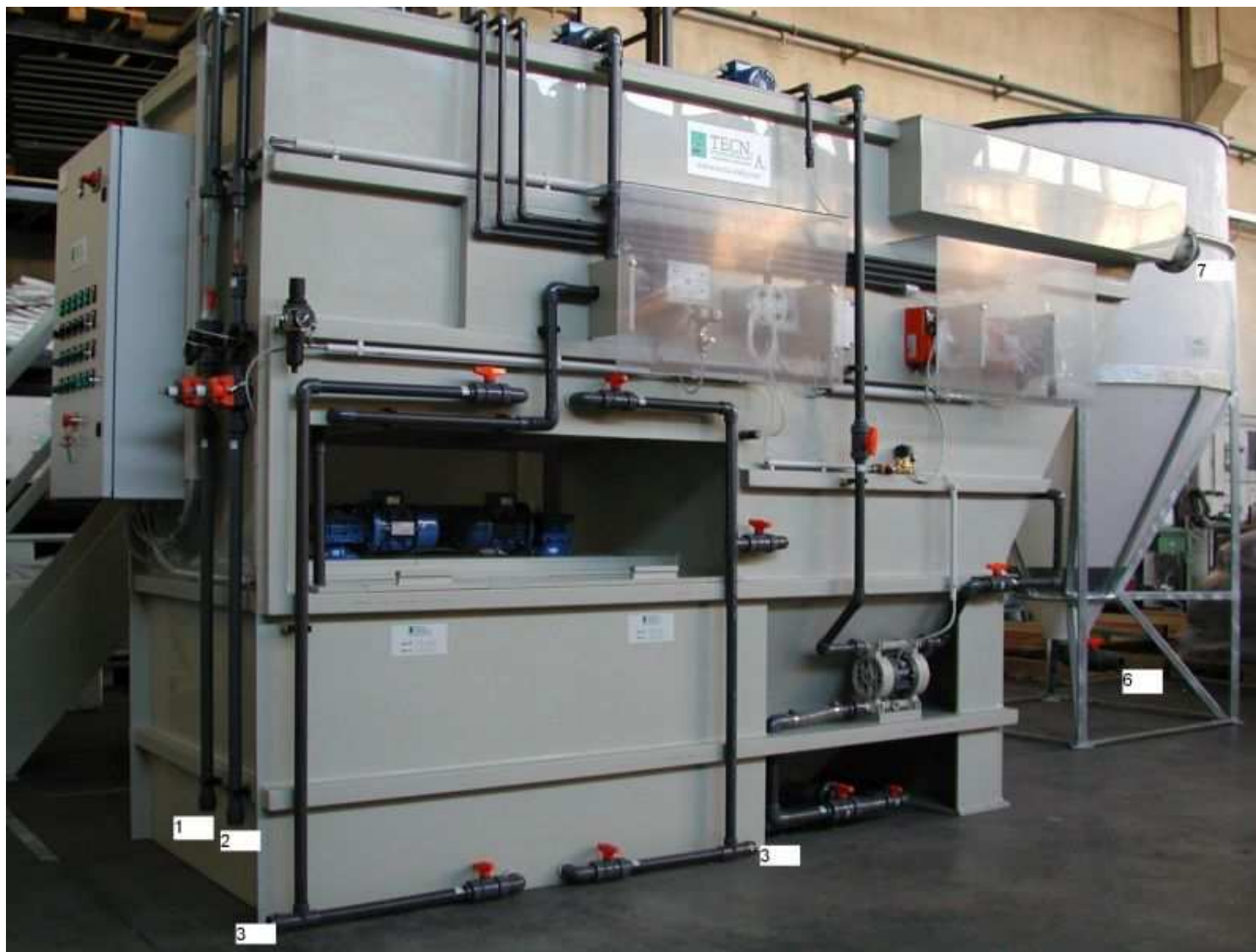
Chemical-physical plant - 2,5 m 3 /h
