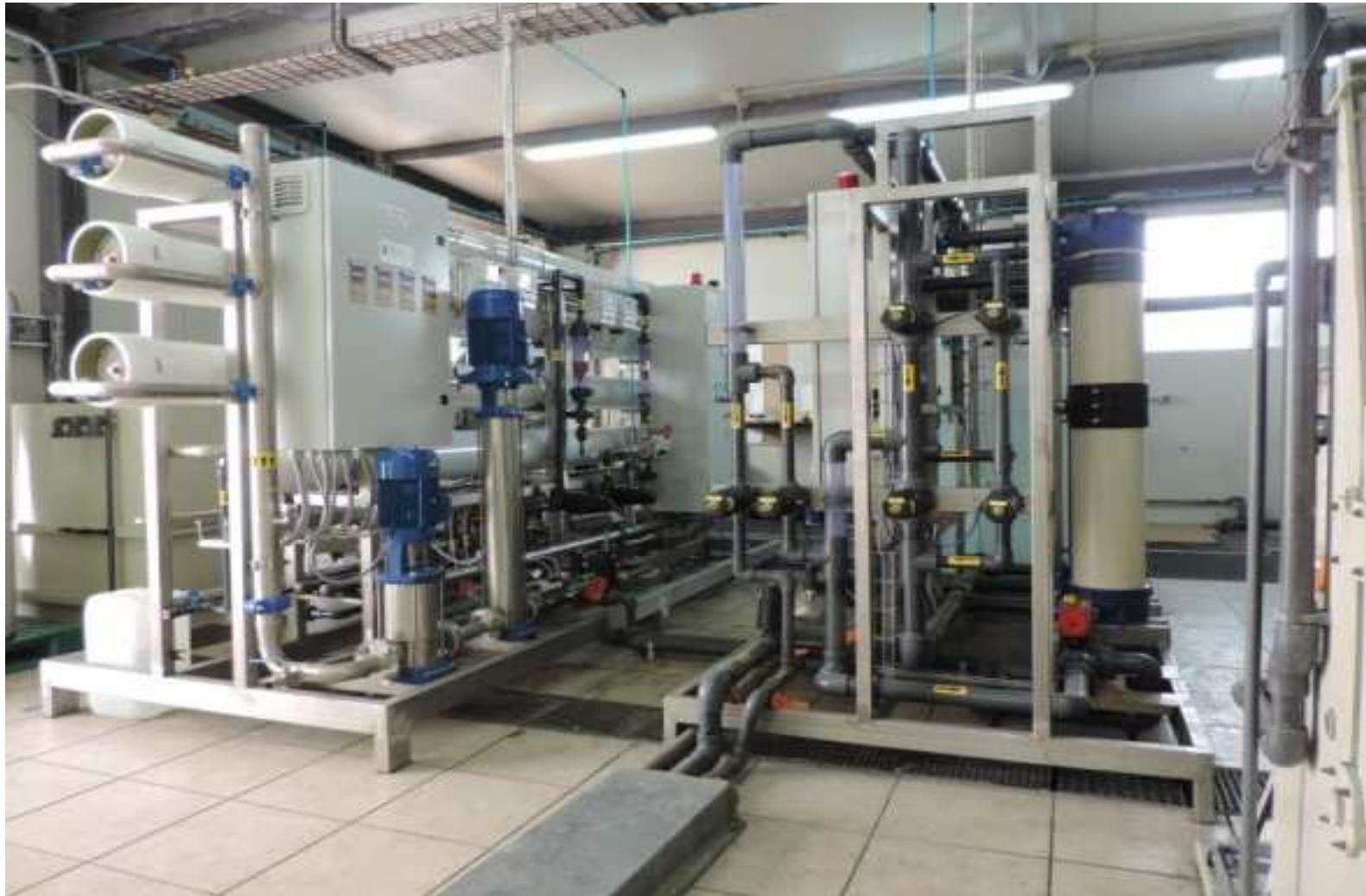
ZLD plant - 5 m 3 /h, with ultrafiltration pre-treatment
