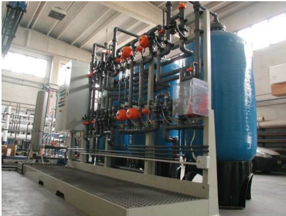
Automatic selective filters - 7 m 3 /h
