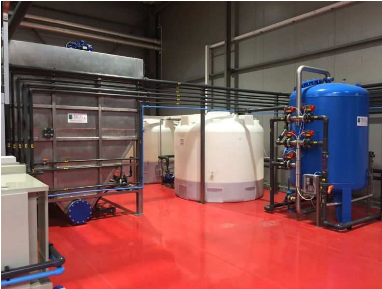
Sand and anthracite filter, with automatic valves, 20 m 3 /h
